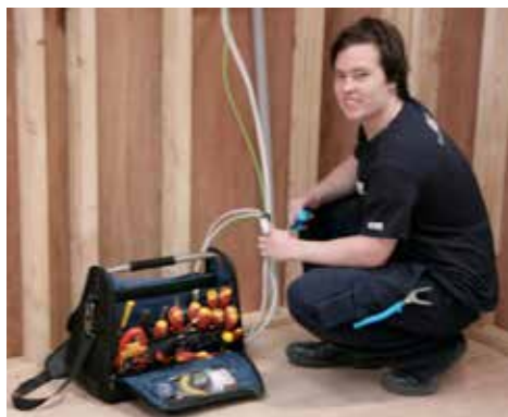
Second-year electrical apprentice Luke Twentyman at work on a transportable houses at Sunshine Campus
